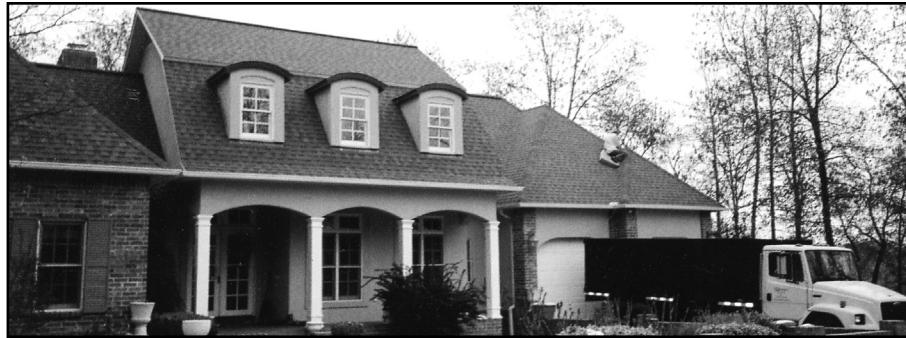
Completion of tear off and replacement job on a home in Flippin, Arkansas.
